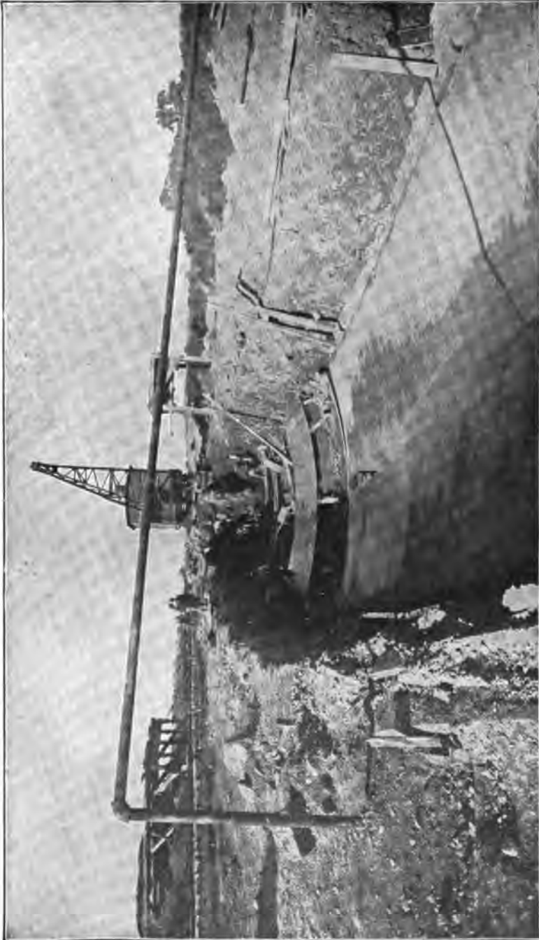
PLATE 134.—Excavating Trench for Cut-and-cover Aqueduct—Firm Earth Section—Using Scraper Buckets. Machine is assisted by gang of men shaping up sides, etc. Concrete invert placed.
